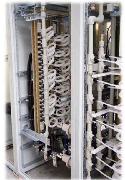
Image courtesy of CKD Elektrotechnika
